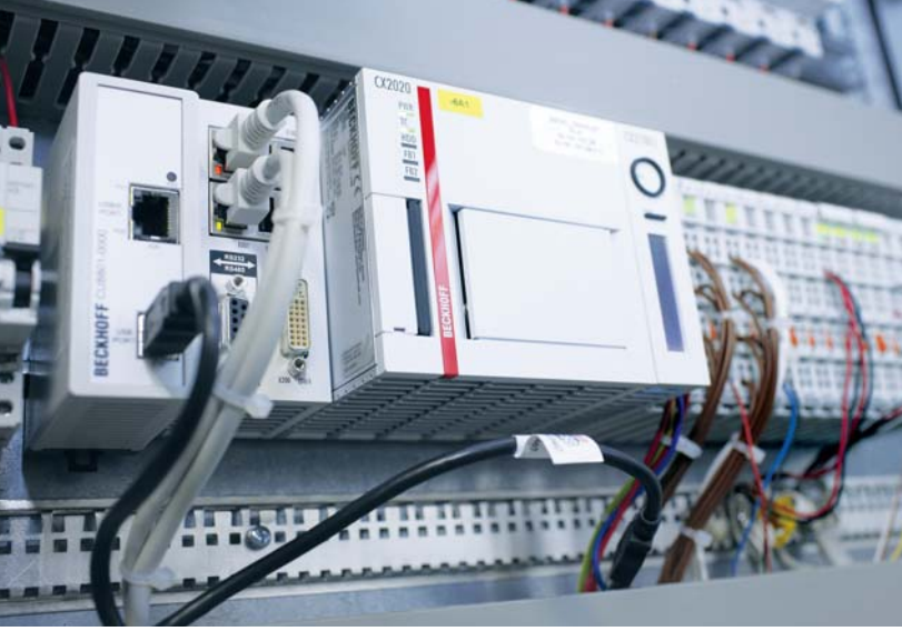
A CX2020 Embedded PC with Intel® Celeron® CPU and a 1.4 GHz clock frequency controls an entire office floor.
