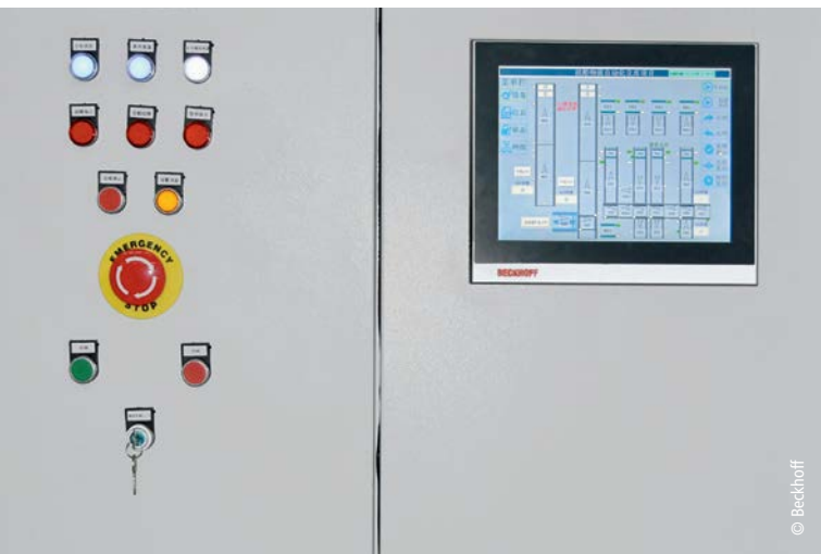
The Embedded PC in the control cabinet is connected to a Beckhoff Control Panel CP2912 used as HMI.
