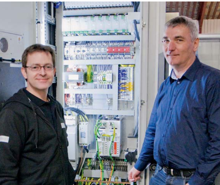
Engineer Bjarne Steenbjerg from Kiermar Technology and application engineer Hans Christian Pallesen from Beckhoff Automation Denmark (from left) in front of the control cabinet of the deep drawing press
