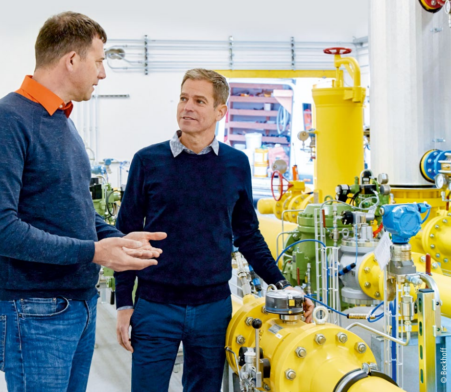
Bertrand Luisier (left), Automation Manager at Gaznat, and Vincent Hauert (right), Beckhoff Branch Manager Yverdon, discuss the advantages of the digitalized gas supply infrastructure.
