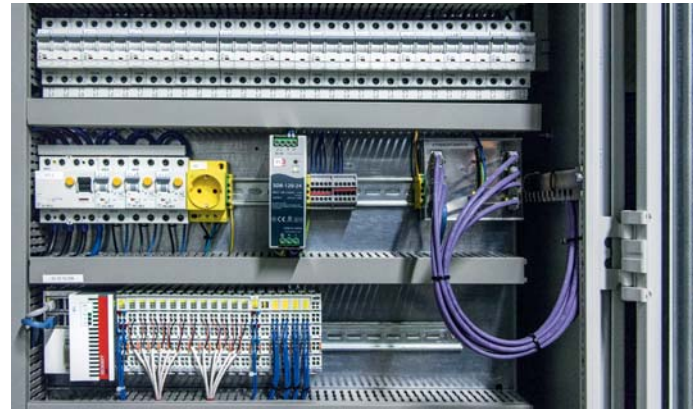
Control cabinet of the LED lighting system with the CX5020 Embedded PC (bottom) and the associated EtherCAT Terminals.
